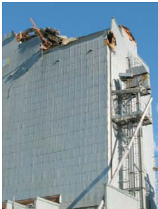
A grain elevator near Brockton hit by microburst winds, July 13, 2005. National Weather Service photo
